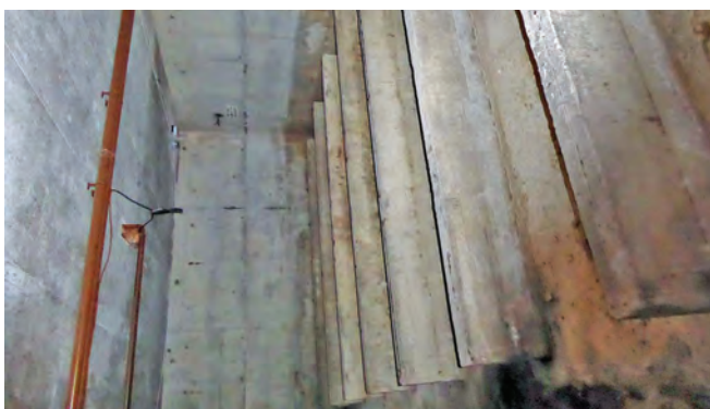
Basement fuel tank room. There was a further room to the left of this, unlit and inaccessible except for a small ‘window’. Photo Julia Shaw
